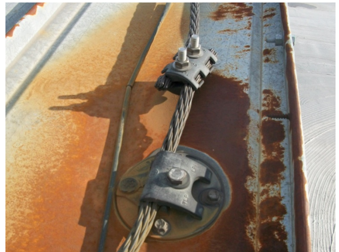
Figure 1: Copper and bronze in contact with galvanized steel.
