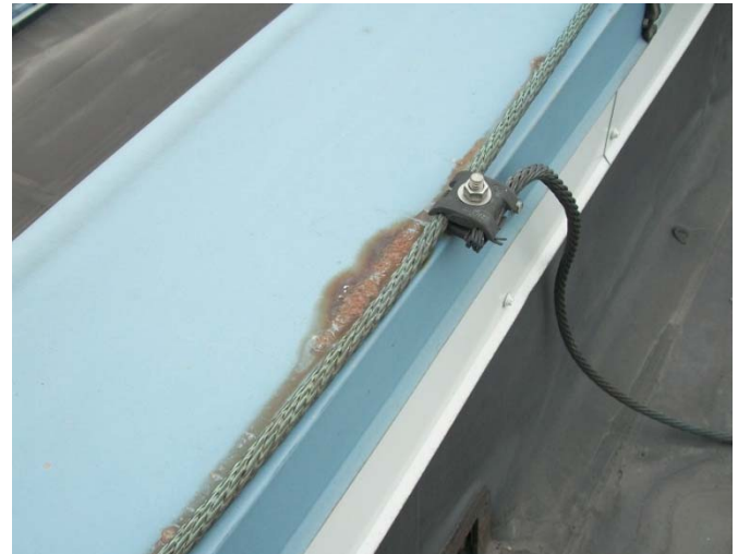
Figure 2: Copper and bronze in contact with painted steel.
