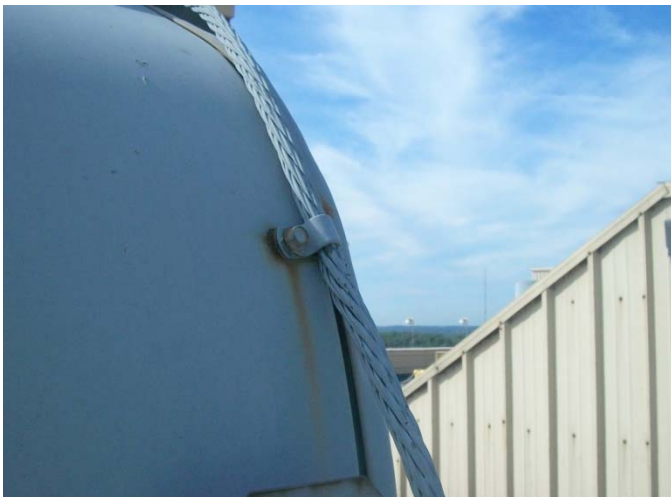
Figure 4: Corrosion between painted unit and painted conductor
