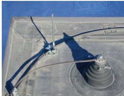
Bonding of metallic bodies and roof components to ensure continuity is a requirement of the lightning protection safety standards.
