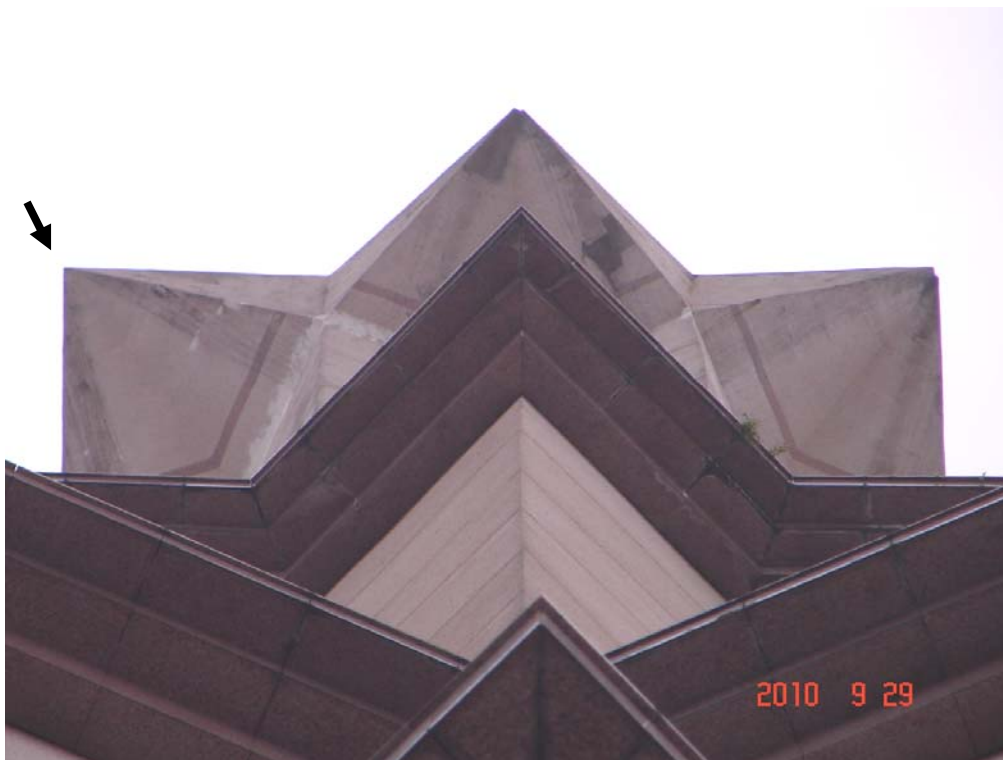
Figure 8: A close-up photo showing three of the concrete protrusions taken from the base of the minaret. Two of the protrusions displayed minor damages while the only remaining undamaged protrusion is shown on the left.
