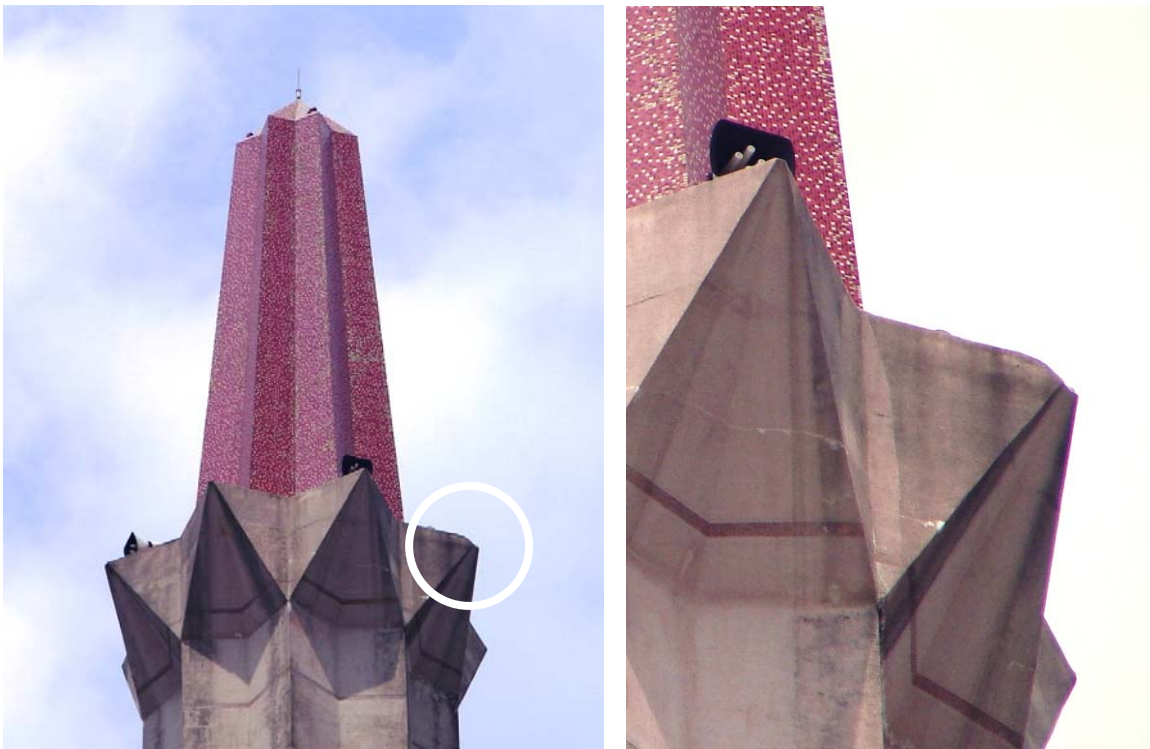
Figure 7: The location of the bypass (left) on the horizontal concrete protrusion and a close-up view of the same bypass (right). Compare this photo with that of Fig. 2 (before the strike). The Helita Pulsar ESE air terminal can be seen on the apex of the minaret about 12 metres above the bypass.
