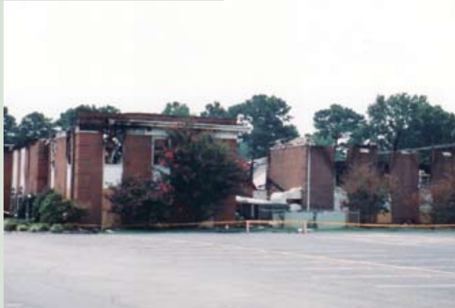
Above: Lightning fires commonly start in the steeple, roof or attic. A direct lightning strike destroyed the entire roof of this church in Mechanicsville, Virginia.
